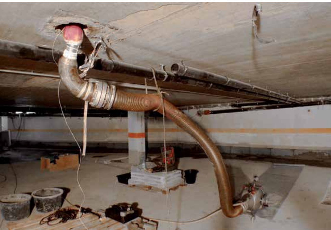
Inversion 7 metres up into the vertical pipe with the epros®Drum type „Mini“
